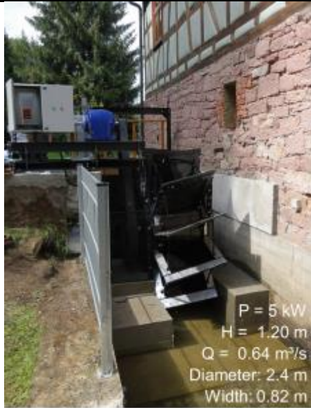
Reactivation of a Mill at Partenstein, Germany with a HPM.
